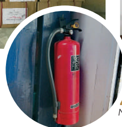
Fire extinguisher in main clinic.
