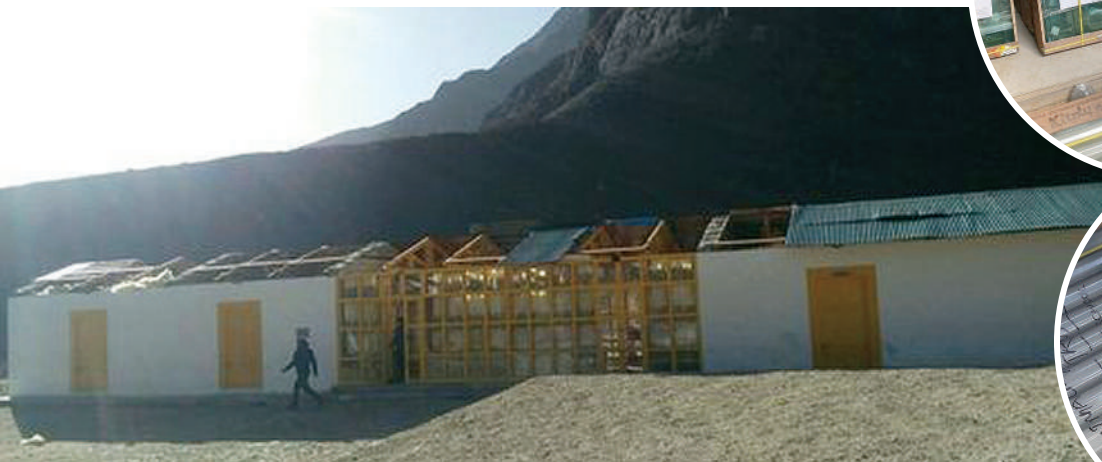
The damaged rooftop of Thame hostel.
